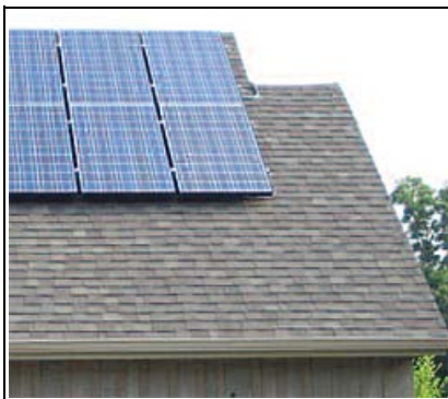
Solar installation at Richard Stumpner's Bloomington home. Photo courtesy Richard Stumpner
