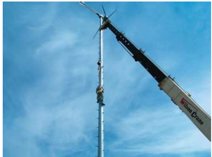
Installation of a wind turbine near Mintonye Elementary School (Photo provided by Eric Cotton, ECI Wind and Solar)
