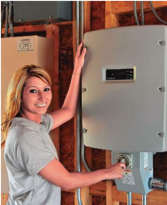
McKenna J Regan, a member of the Purdue Solar Decathlon team, stands next to the solar house service panel.
